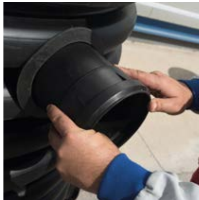
A plastic adapter is inserted to connect the pipe to the manhole.
