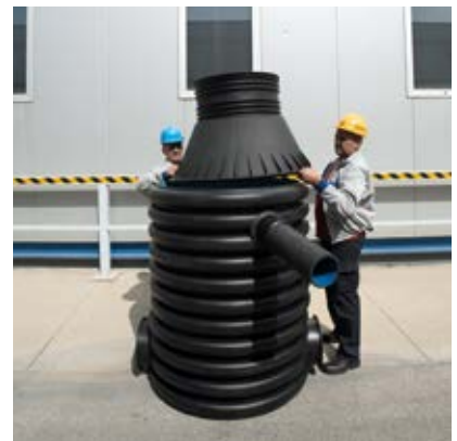
The installation of the cone and the manhole is ready for the final internal welding of all joints.
